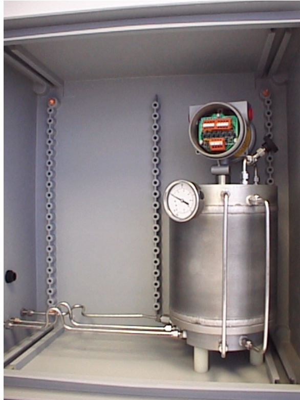
Figure 1-1 View of the 3098 specific gravity meter installed in a typical enclosure
